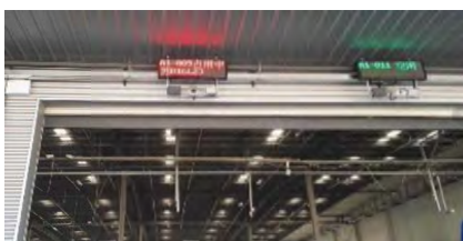
Dock Management System
